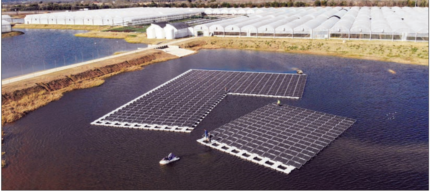
During installation, workers use personal watercrafts to maneuver parts of the array into position. Photo courtesy of Speir Commercial & Industrial
