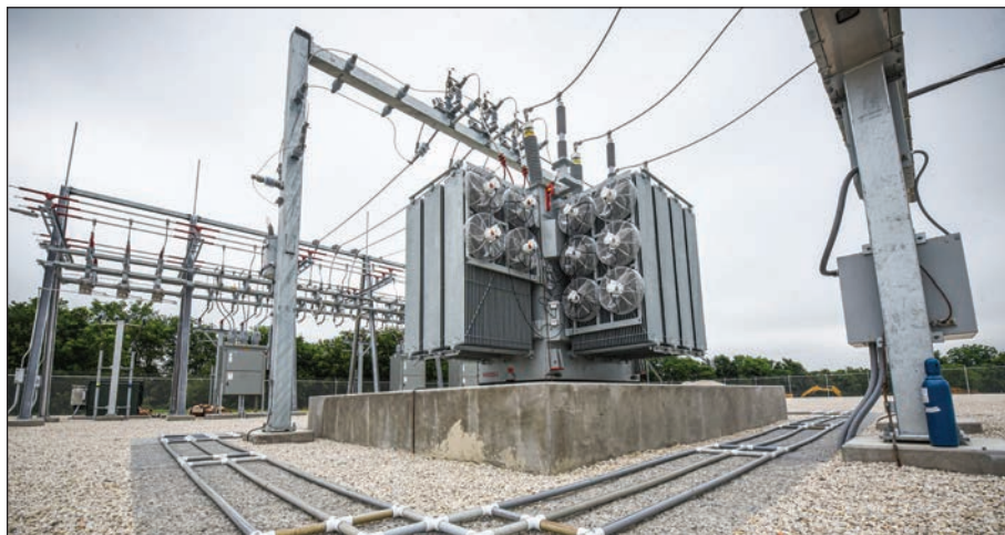
The new Cooks Point substation, above. Below, substation technicians Brian Seymour, at left, and Michael Gholson installed the wiring in the facility outside of Caldwell.
