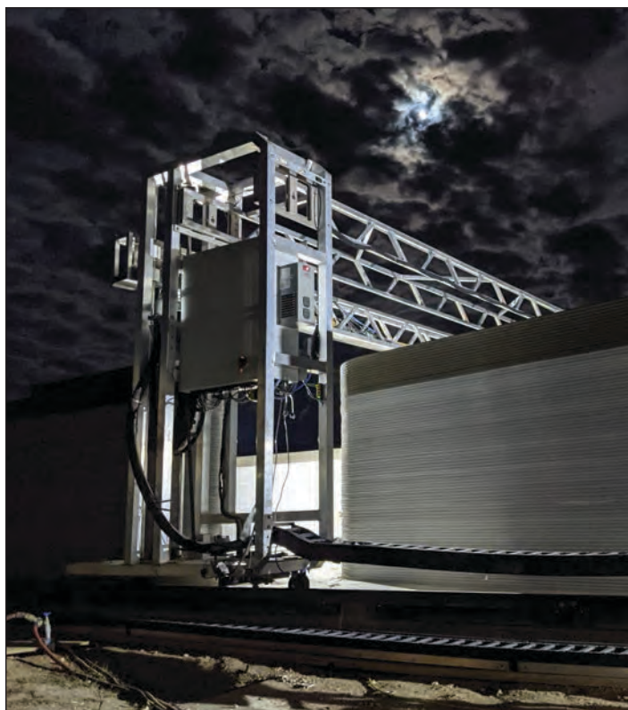
The massive 3D printing machine at work, creating the walls of a barracks at Camp Swift. The machine weighs 9,500 pounds and can print a wall up to 10½ feet high. ICON photo
