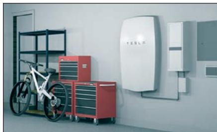
Battery storage units like the Tesla Powerwall can save your solar array's overproduction. Photo courtesy Tesla Motors, Inc.
