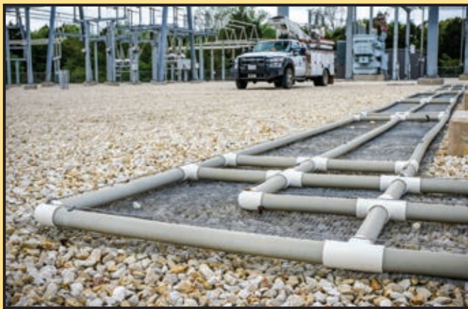
If a snake manages to get past the barriers outside a substation, it still has to contend with electrified wires between PVC pipes that surround equipment. (Sarah Beal photo)
