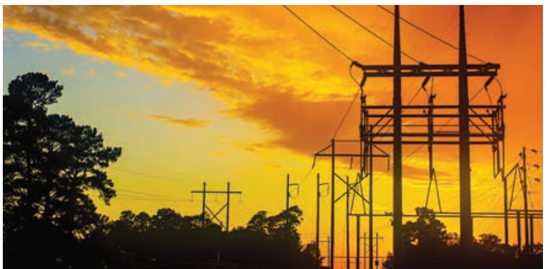
▼ MARK HUSFELD , Navasota Valley EC: Near a substation in Navasota after a thunderstorm.
