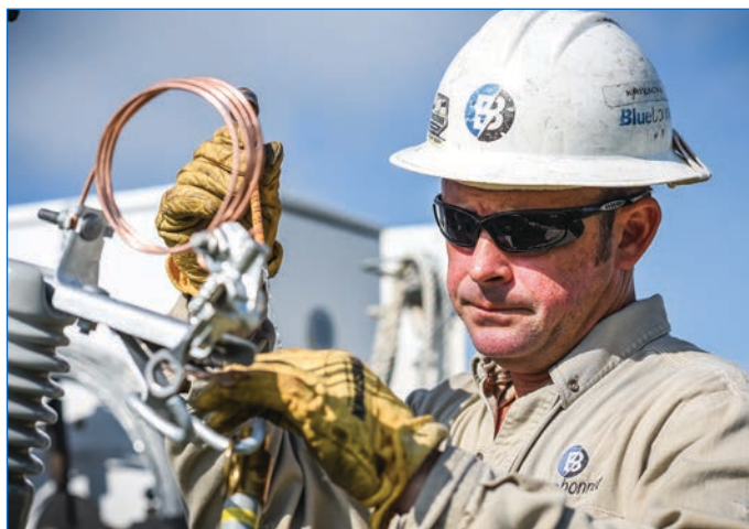
Check Bluebonnet's social media on April 11 for a tribute to our line workers. Here, Brandon Krivacka, in Brenham, prepares a transformer to be installed at a location where new construction is taking place. Sarah Beal photo
