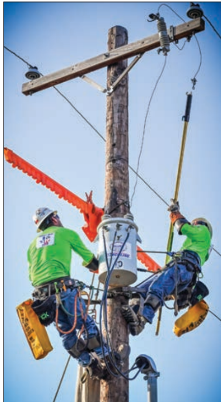
Troy Moore and Kendal Fiebrich compete in the transformer change-out event.
